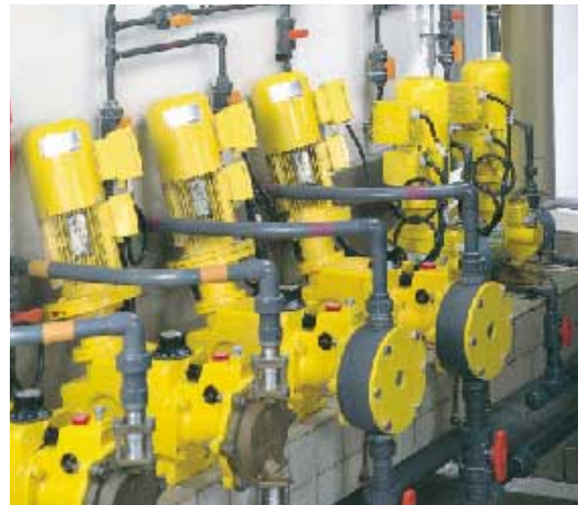
Water treatment : MAXROY® pumps in effluent treatment plant.
