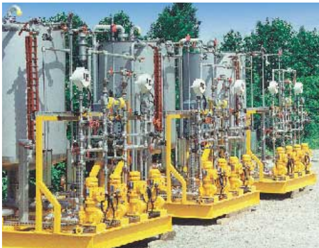
Oil industry : Corrosion inhibitor injection package for oil treatment.
