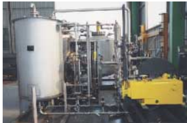
Oil and Gas industries : Dosing packages for sulphuric acid, caustic soda, dimethyldisulfide in a refinery subjected to severe atmospheric conditions.
