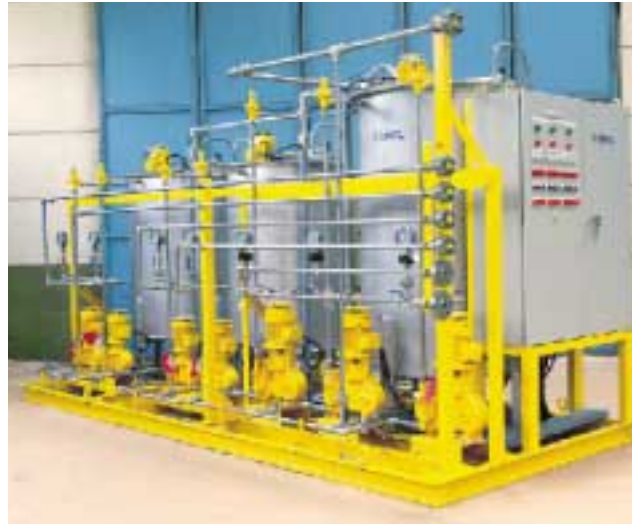
Water treatment : Preparation and dosing of hydrazine and phosphate for boiler water treatment.
