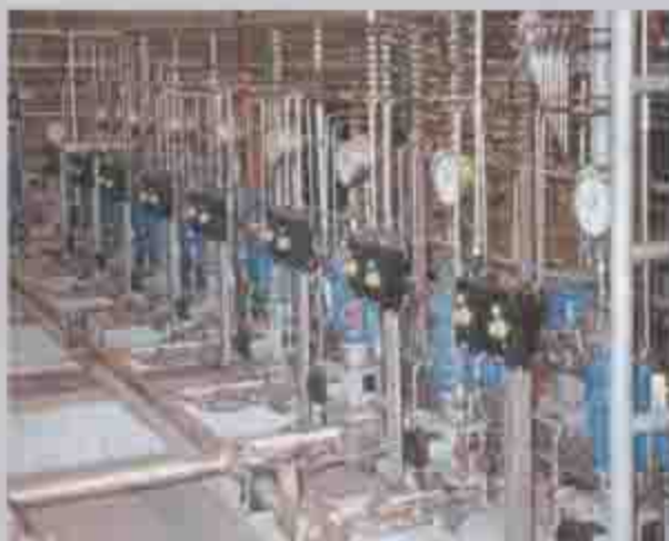
Typical Multi-Pump System with numerous pipe runs and large skid obstructing direct access to the pumps. The increased number of pumps leads toward increased maintenance, larger and more expensive construction.
