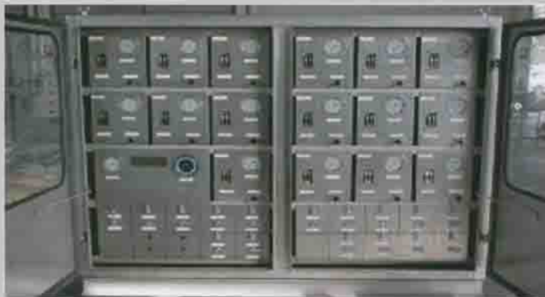
Typical Haskel IRCD panel injecting chemical into 16 injection points, utilizing only one small pump and one square. Note the apparent ease of operation and layout.
